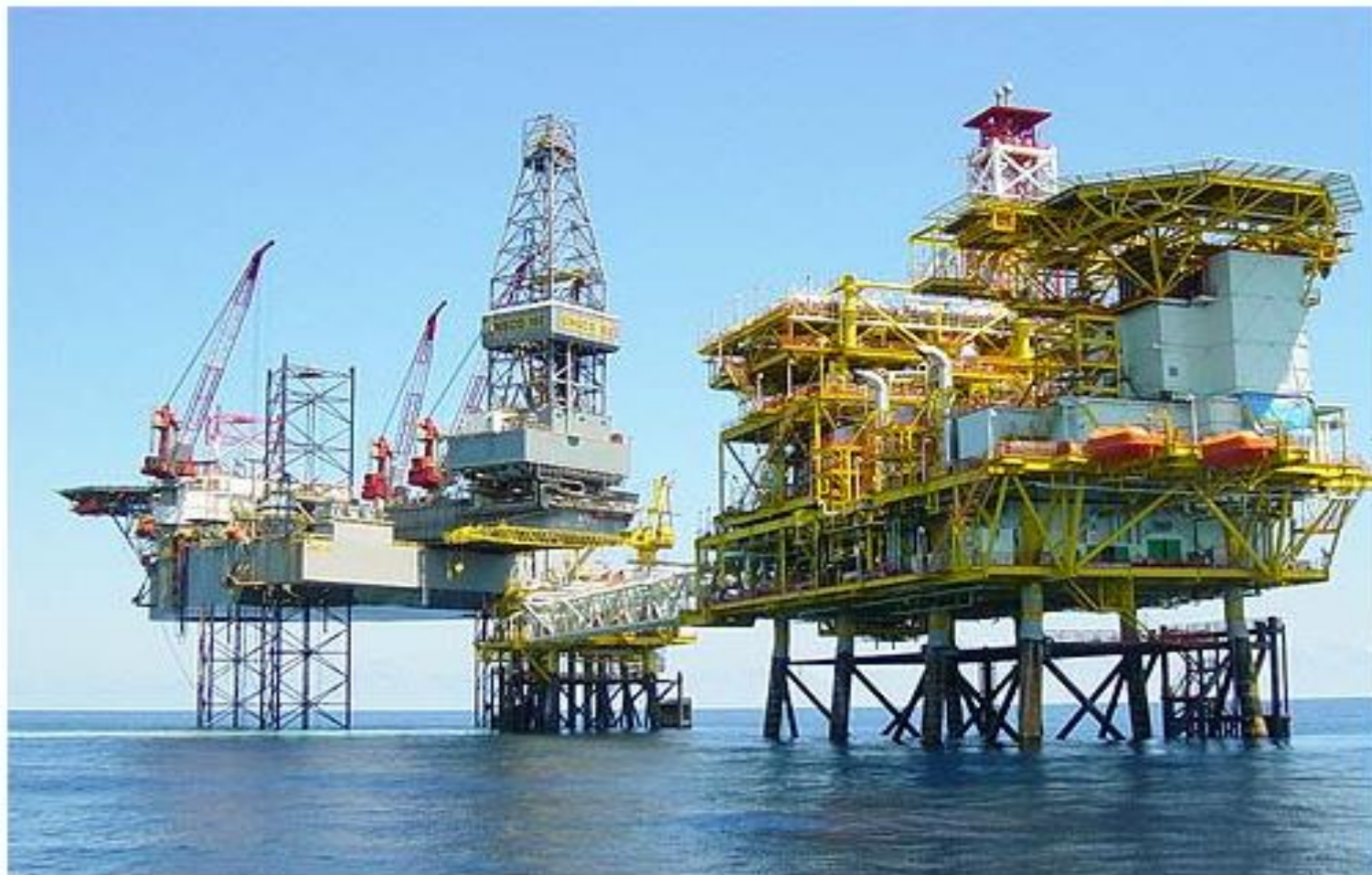
Petronas/Shell B11 Platform - First commercial application of the revolutionary Twister Supersonic Gas Processing technology.
