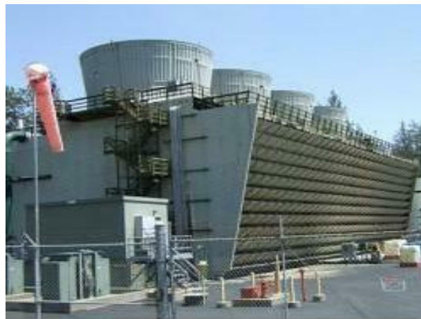
Industrial cooling tower
